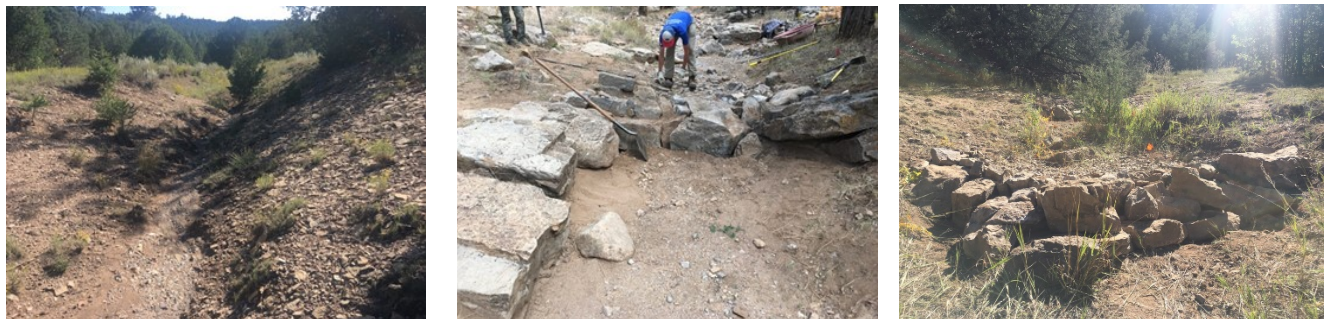
Figure 17. Bank erosion (left), structure installation (center), and installed structures (right). Photo credit: Rocky Mountain Youth Corps/Stream Dynamics, 2019
