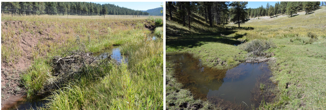
Figure 21. Images showing work completed by 2023. Image (left): BDA installation, with exclusion fencing at top of slope; Image (right): An installed BDA, demonstrating the additional ponded area behind BDAs
