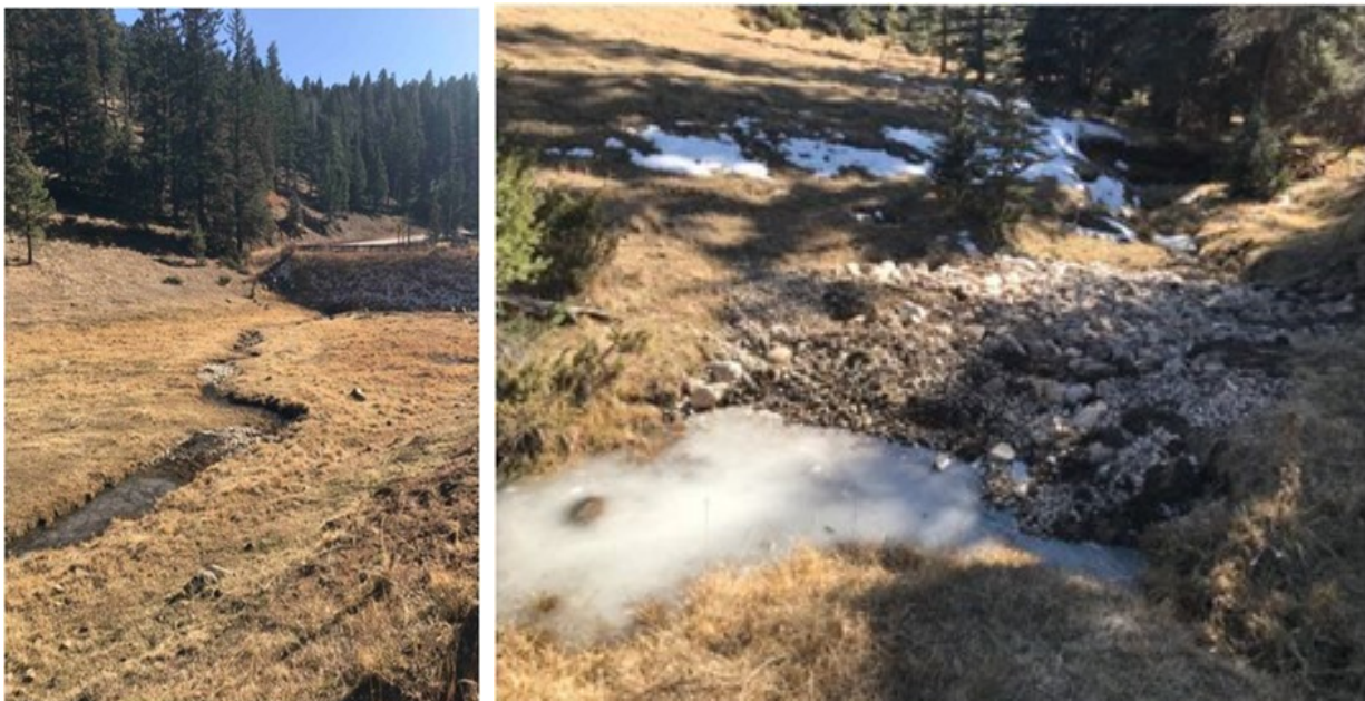
Figure 15. Left: Lower project area restoration structures (3 visible in photo). Right: Headcut repair and erosion control at project site. Photo credit: Rachel Conn, Amigos Bravos, 2019.
